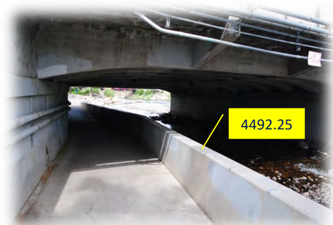
Figure 4. Existing Path and Solid Barrier under North Bridge
