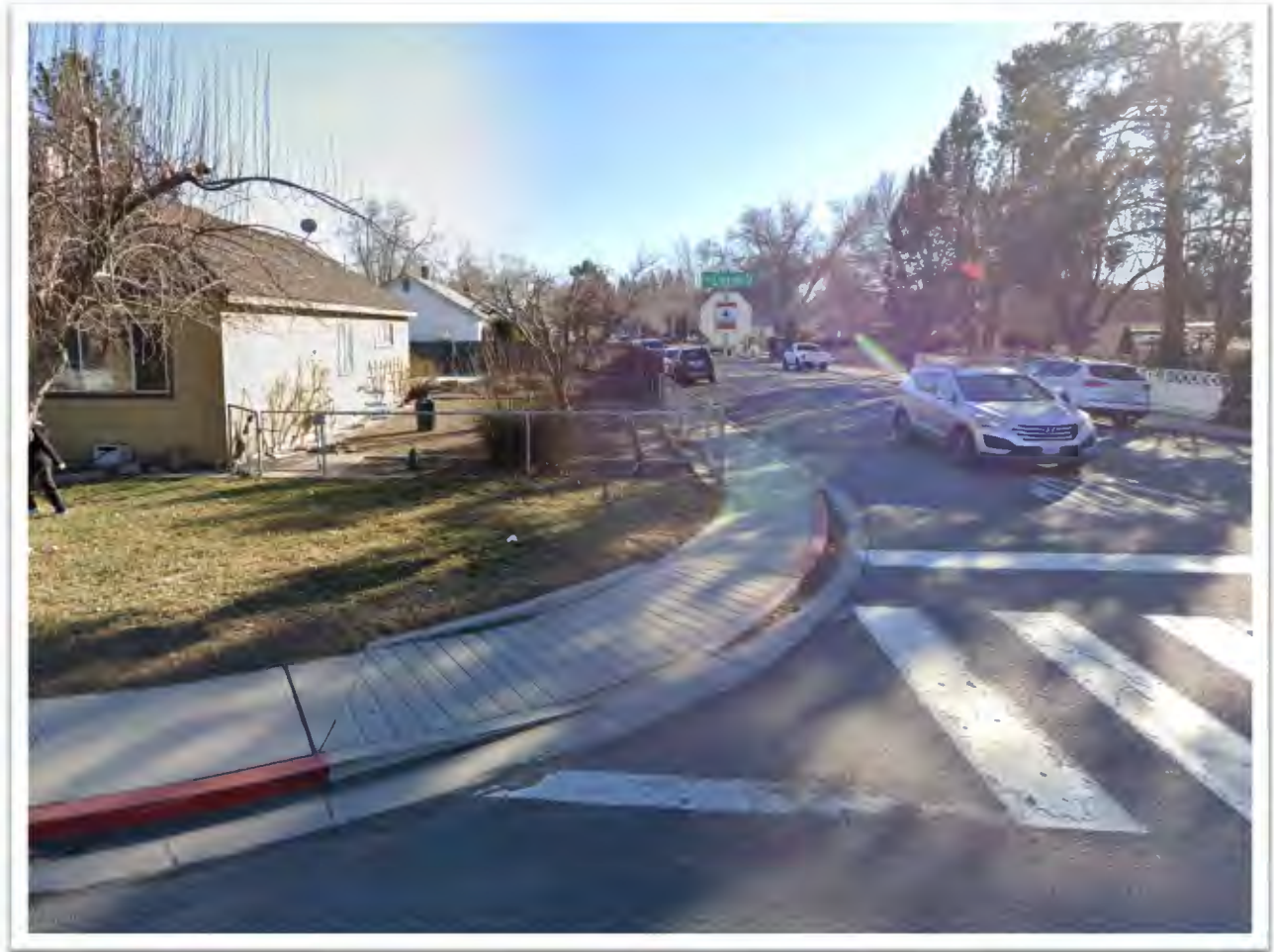
Example of an Existing Non-Compliant Pedestrian Ramp
