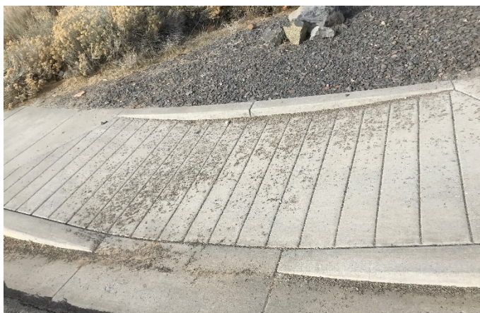
Figure 5.21: Non ADA Compliant Ramp @ Calle de la Plata
