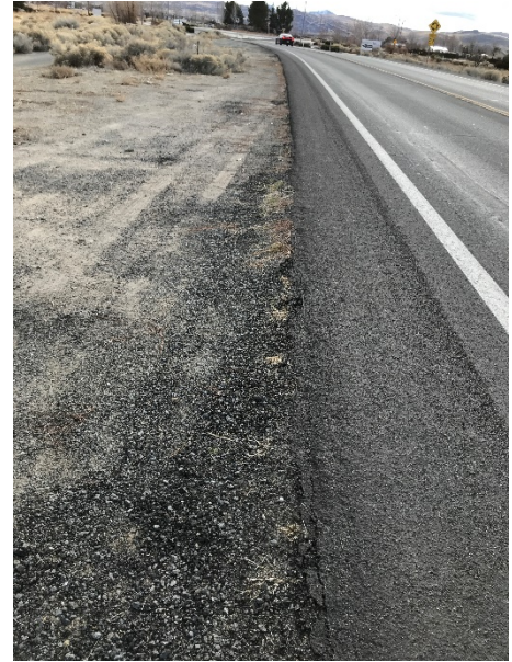
Figure 5.18: Eagle Canyon Drive Pavement Shoulder along Shaw Middle School
