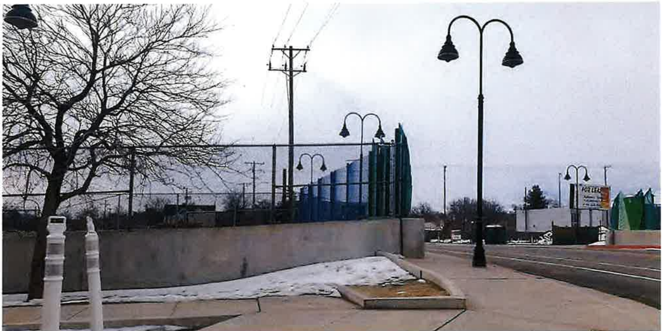
The existing train trench wall presents a potential sight distance issue for bicyclists and pedestrians crossing major streets
