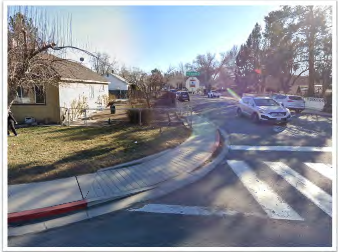
Example of an Existing Non-Compliant Pedestrian Ramp
