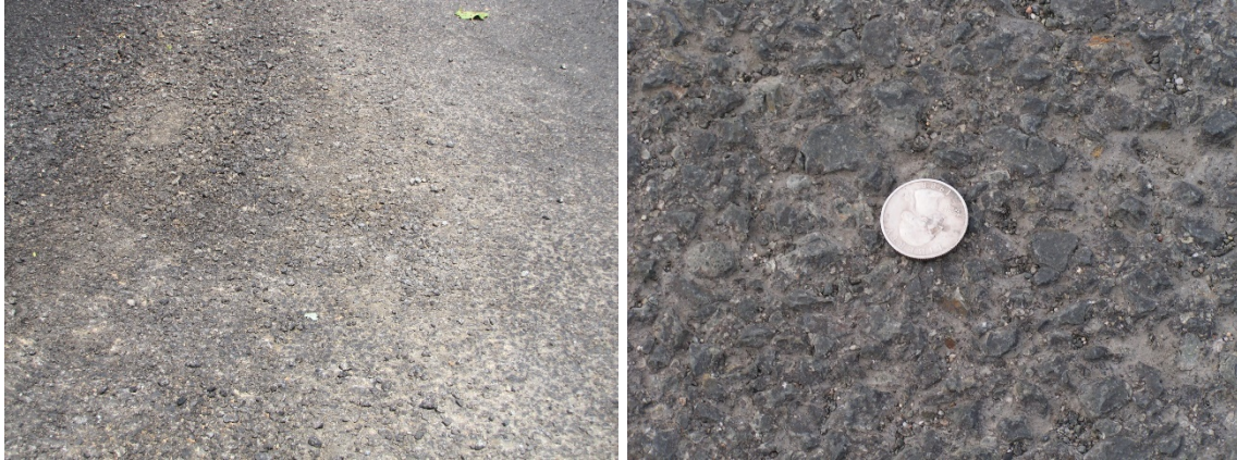
Figure 13. Typical raveling of flexible pavements in northern Nevada.
