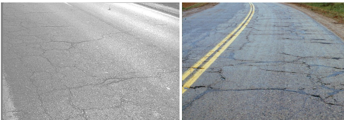
Figure 12. Typical block cracks in flexible pavements in northern Nevada.
