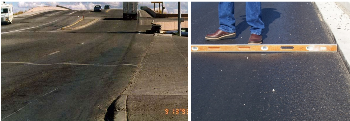
Figure 7. Typical wide ruts formed in the base, sub-base, or subgrade layers.
