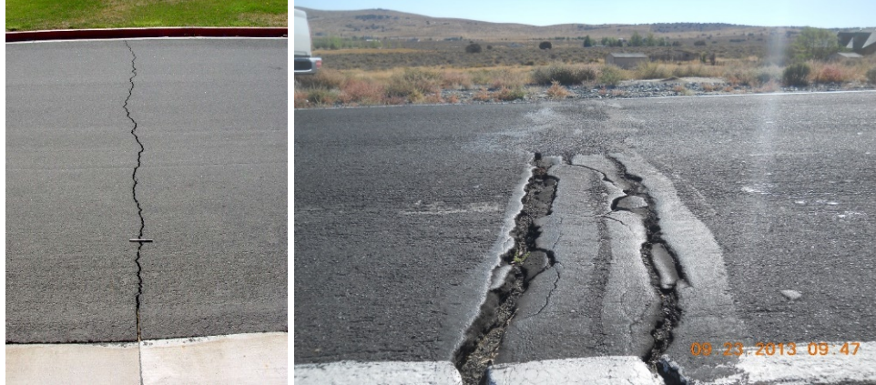
Figure 11. Typical transverse cracks in flexible pavements in northern Nevada.
