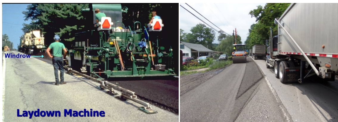
Figure 24. The CIR mix is picked up by the paver and roller compacted.
