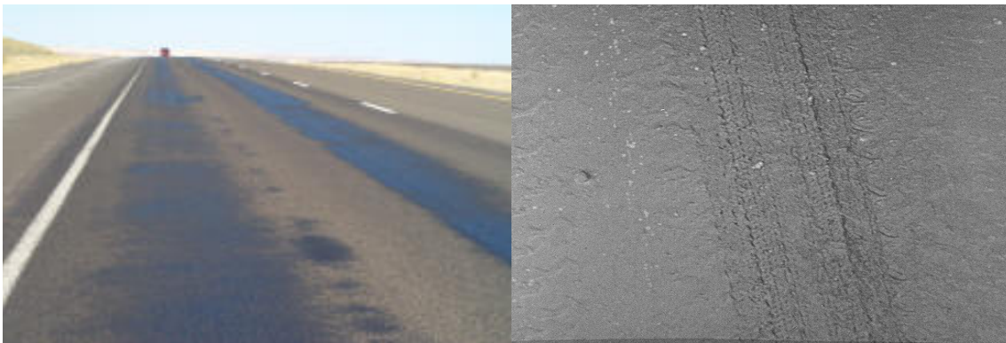
Figure 9. Medium and severe bleeding failures of flexible pavements.
