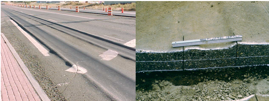
Figure 6. Typical narrow ruts formed in AC layer.
