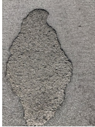
Figure 14. Typical functional pothole on surface treatment.
