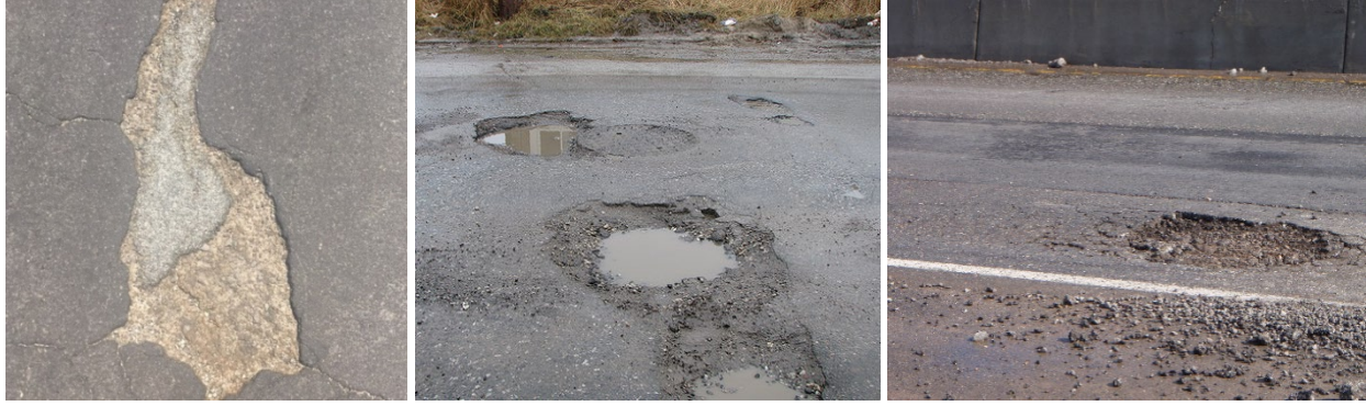
Figure 15. Typical structural potholes.
