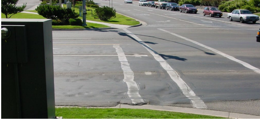
Figure 5. Typical shoving of flexible pavements.
