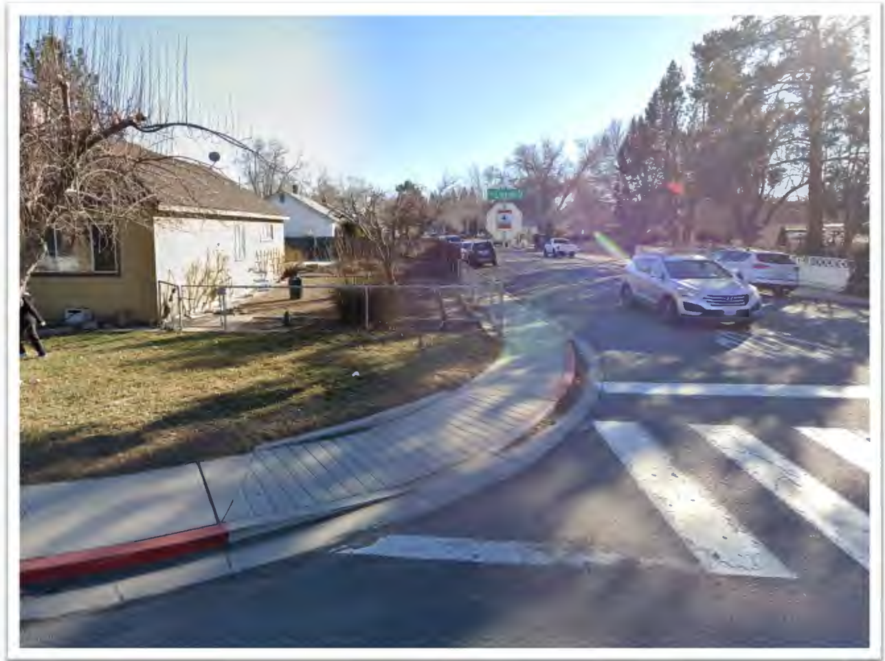
Example of an Existing Non-Compliant Pedestrian Ramp
