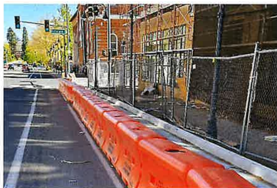
Figure 6.6 Water-filled barriers on Arlington Ave which can be used for quick-build installations.
