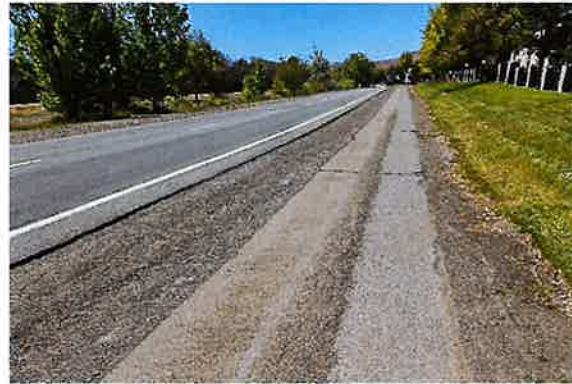
Figure 6.1 Local shared-use path with significant dirt build up.
