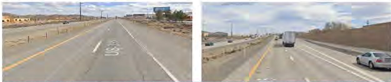
The project will fully reconstruct US 395 that is deteriorating and cracking. (Source: Google Maps, 2021)
